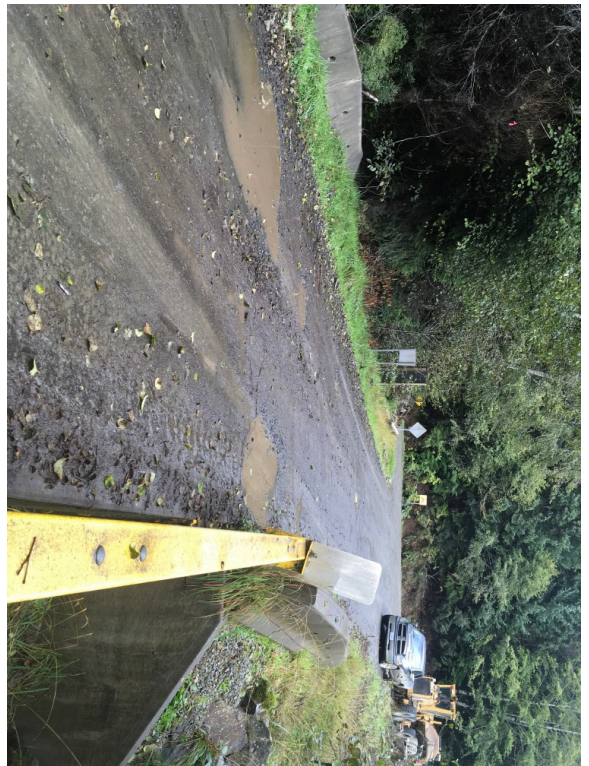
Leaning concrete no posts on left abutment.
