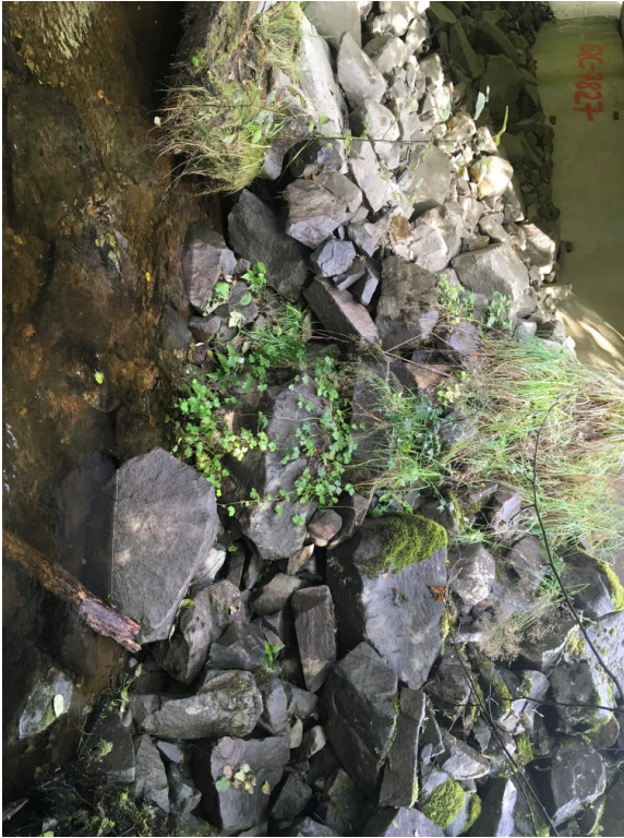
Riprap actively being scoured.
